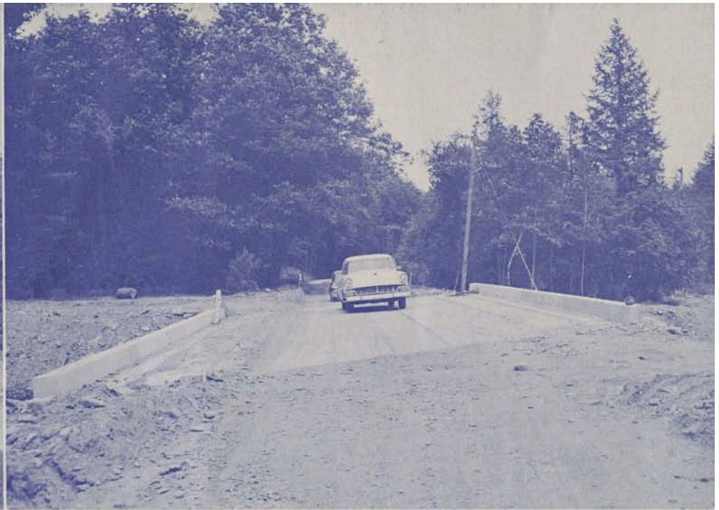
POCONO CREEK, east of Tannersville. Legislative Route 45024. Concrete beam span 74 feet to replace concrete bridge.
