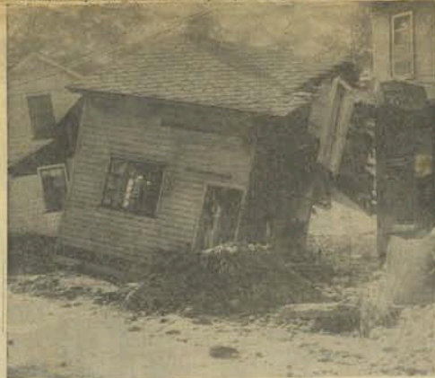
The fury with which flood struck Moosic, south of Scranton, is evident from the way this house was torn apart and swept from its foundations.
