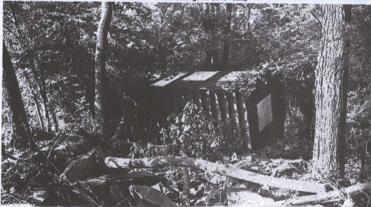
1955 Flood Damage at Girls' Camp
